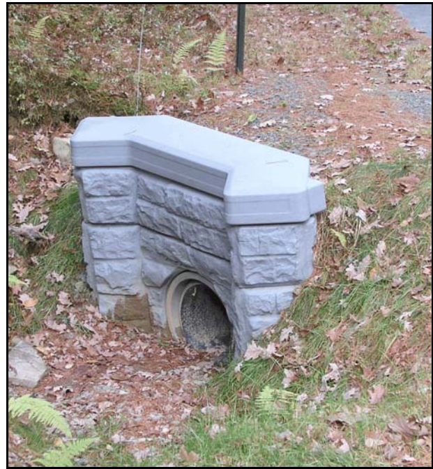
Plastic Culvert / Plastic Head Wall, Spring Road
